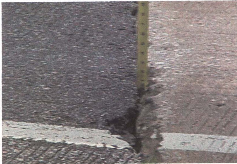
PAVEMENT SETTLEMENT AND RAVELING 'B' APPROACH
