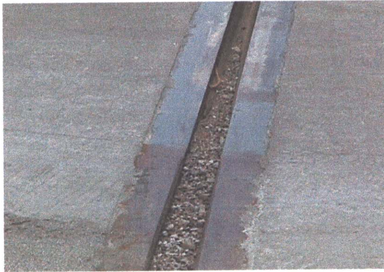
LIGHT DEBRIS AT JOINT
