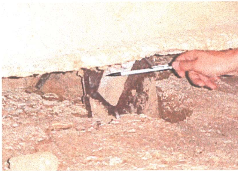
CORROSION ON PILES ABUTMENT #1 TYPICAL
